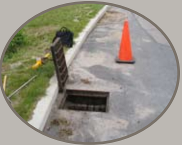
Leaching Catch Basins
